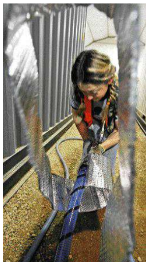
Richelle Klyne wraps a hose with bubble wrap at Seair on Monday.
